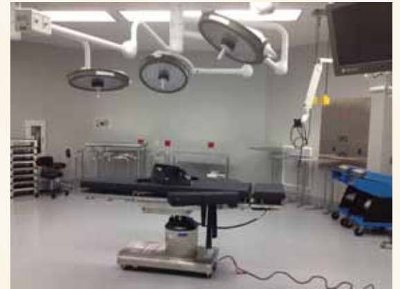
Flowers Hospital recently completed a $3.7 million expansion project to add two additional operating rooms to the Surgical Services Department.
